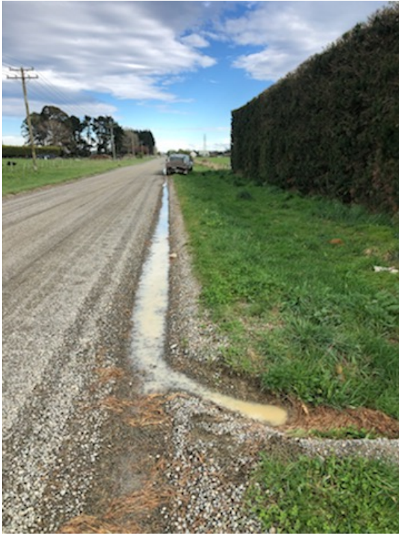
Figure 2: Fine sediment run-off from gravel into drain (river-sourced gravel) – Marsh Road September 2021
