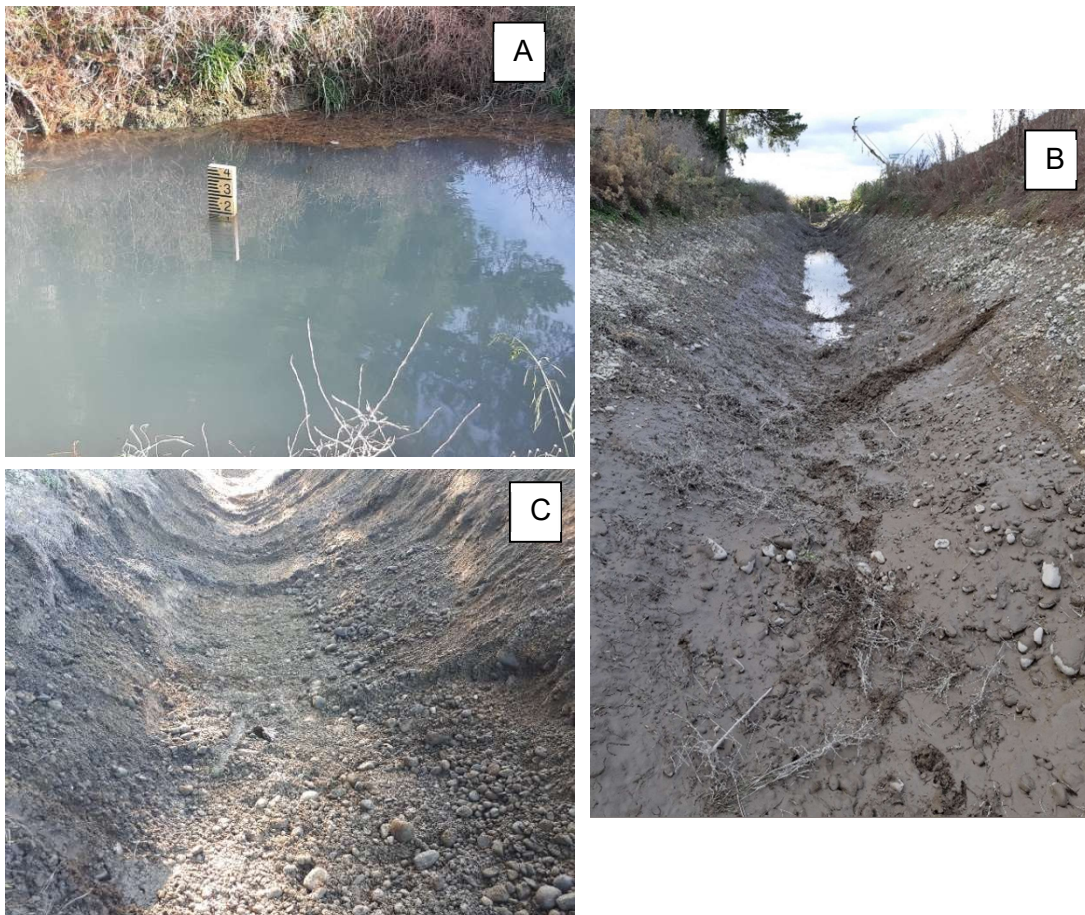
Figure 11 Photo A – Water in the trench has high turbidity. Photo B – The bottom of the trench after a quick clean with a digger while water was still standing in the trench. Photo C – the bottom of the trench after being thoroughly cleared by a digger during dry conditions
