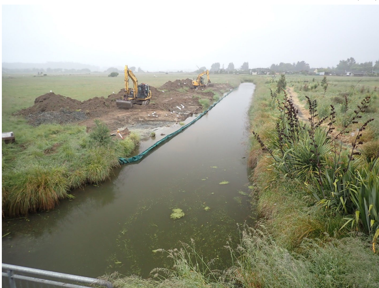
Figure 1: Rebattering earthworks on the True Right of the Taranaki Stream at the floodgate, for improved īnanga spawning habitat.
