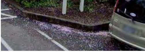
Bad kerb &amp; channel
