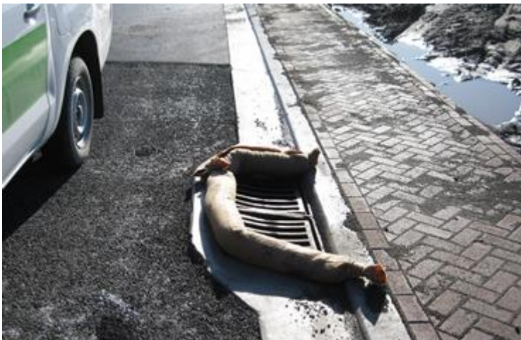
Figure 2. Silt socks installed around the sump to protect contaminants from draining inside it.
