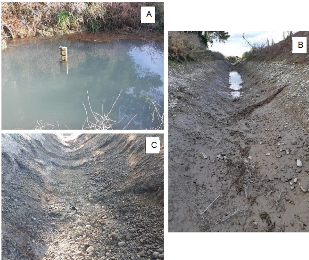
Figure 11 Photo A – Water in the trench has high turbidity. Photo B – The bottom of the trench after a quick clean with a digger while water was still standing in the trench. Photo C – the bottom of the trench after being thoroughly cleared by a digger during dry conditions
