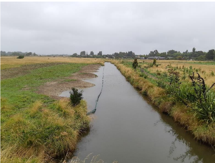
Figure 2: After completion of earthworks, January 2022. The spoil piles are located to the far left of the image, well back from the edge of the waterway.
