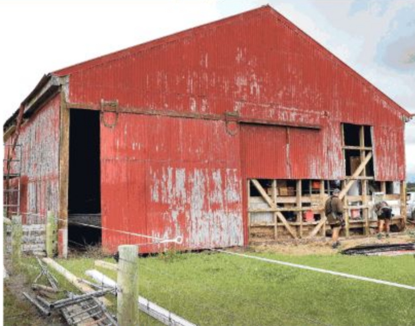
New life . . . Work continues on the almost 150-year-old former railway goods shed at Springbank.
