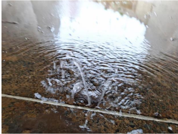
Figure 5: repaired joint with groundwater spouting through
