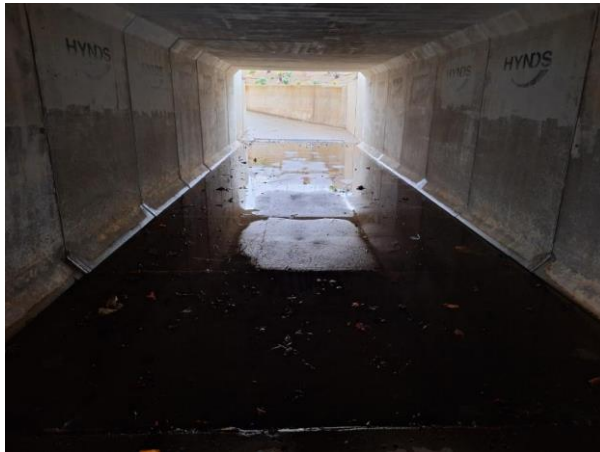
Figure 6: looking through the underpass towards Bellgrove – water evident throughout
