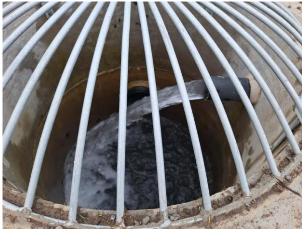
Figure 8: outlet of the groundwater pump into the SMA scruffy dome; pipe full
