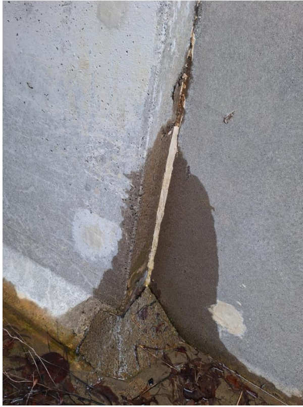
Figure 7: leaking joint at entrance to underpass
