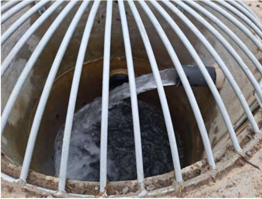
Outlet of underpass pump into Bellgrove SMA
