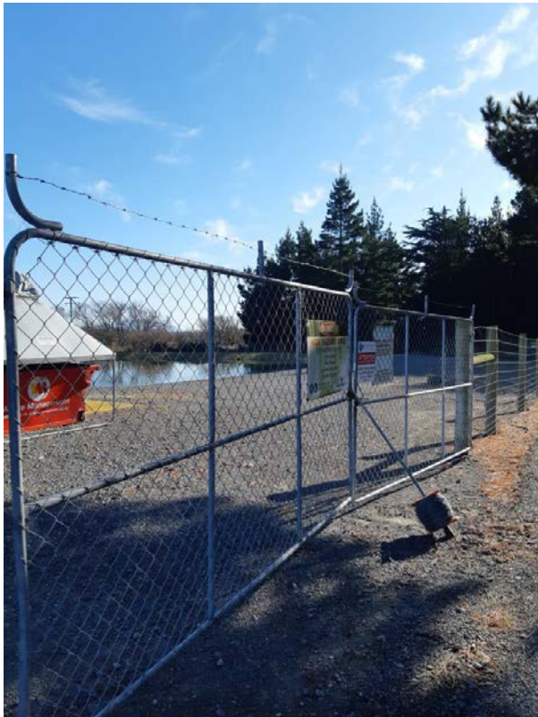
Figure 4: Barbed Wire installed at the Waikuku WWTP site above the entrance gates.
