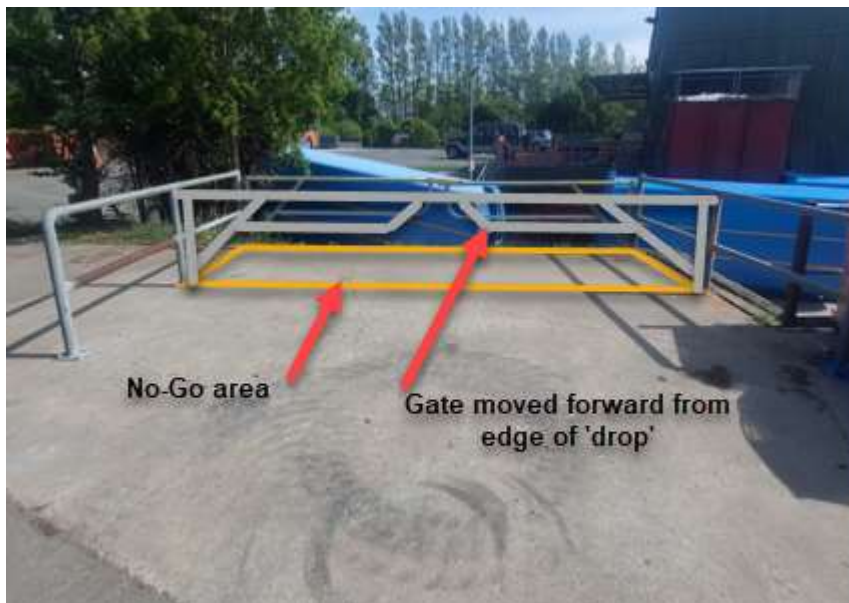
Figure 4.2: Scrap Steel drop-off at “saw-tooth” with fall protection and ‘no-go’ demarcation.
