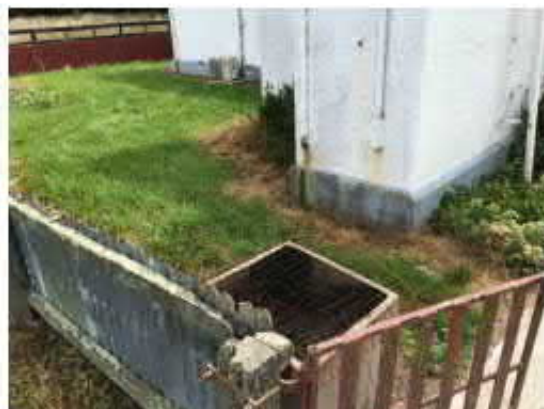
Figure 4: Concrete bin that appears to have been used to incinerate domestic rubbish. It is not known where potentially contaminated ash has been deposited.
