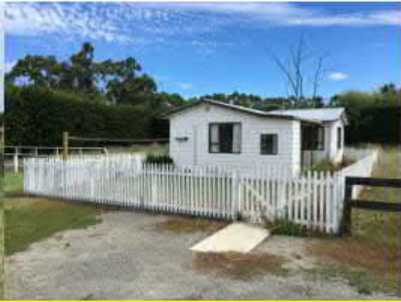
Figure 8: More recent residential dwelling, established in the 1980s. The exterior cladding and internal plaster materials might contain asbestos fibres.
