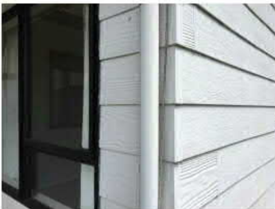
Figure 9: Exterior cladding of the more recent residential dwelling (possibly containing asbestos).
