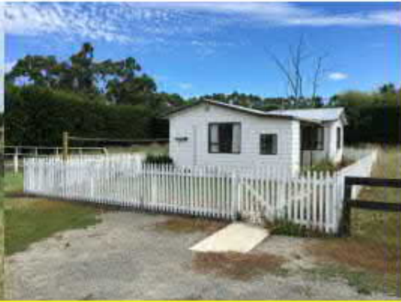
Figure 8: More recent residential dwelling, established in the 1980s. The exterior cladding and internal plaster materials might contain asbestos fibres.
