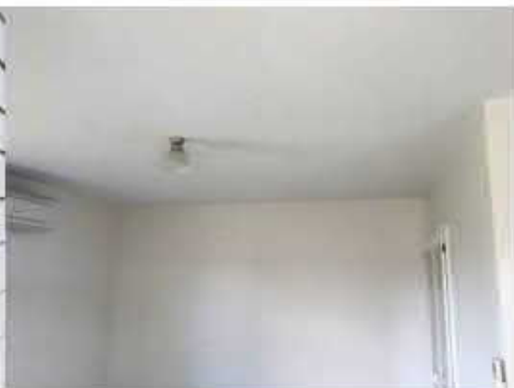
Figure 10: Stippled ceiling plaster in the more recent residential dwelling (possibly containing asbestos).
