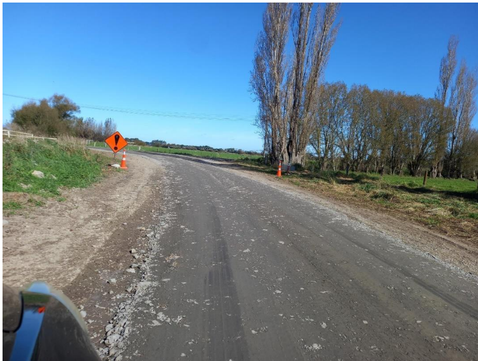
Figure 7: A trial argillite roading section on Waikoruru Road, in the approach to the bridge over the Cam River. Note the argillite has created a hardened surface that prevents erosion of the material and dust into the waterway.
