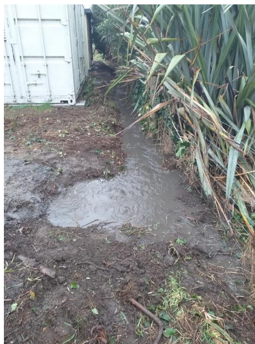
Figure 7. Kings Avenue downstream bubble-up sump opposite 37 / 39 Kings Avenue, and drainage path to the north behind the water pump station.
