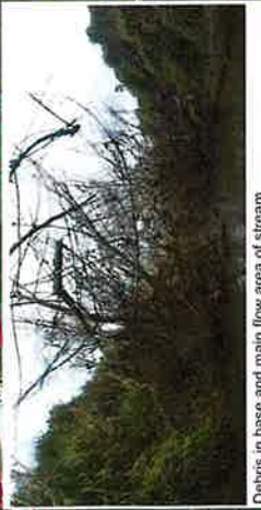
Tree down in main flow area - significant blockage
