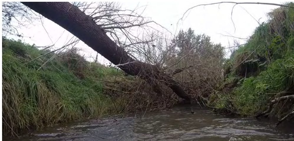
Figure 2- Fallen Tree observed from maintenance inspection.
