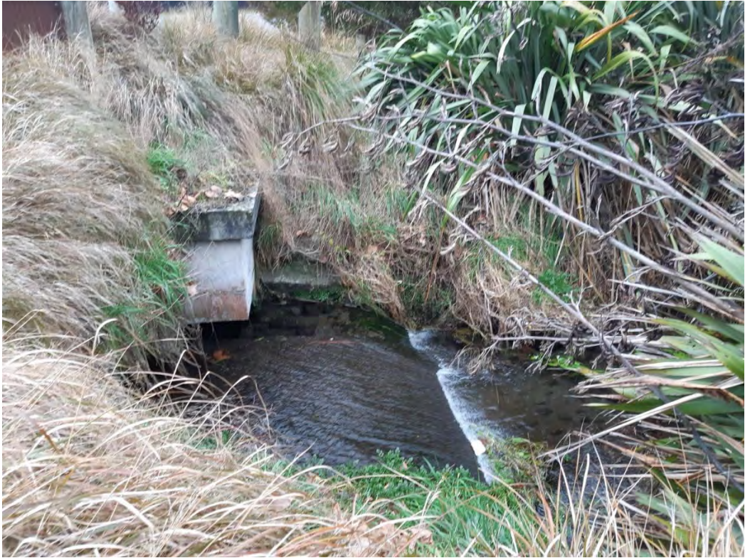
Figure 1: Likely partial fish passage barrier on a North Brook tributary – Corner of Cotter Lane and Northbrook Road
