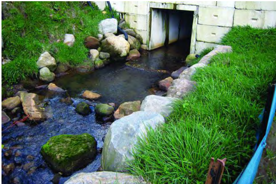
Figure 2: A rock ramp constructed to enable fish passage through a culvert by creating a pool downstream. (Photo credit: NIWA)
