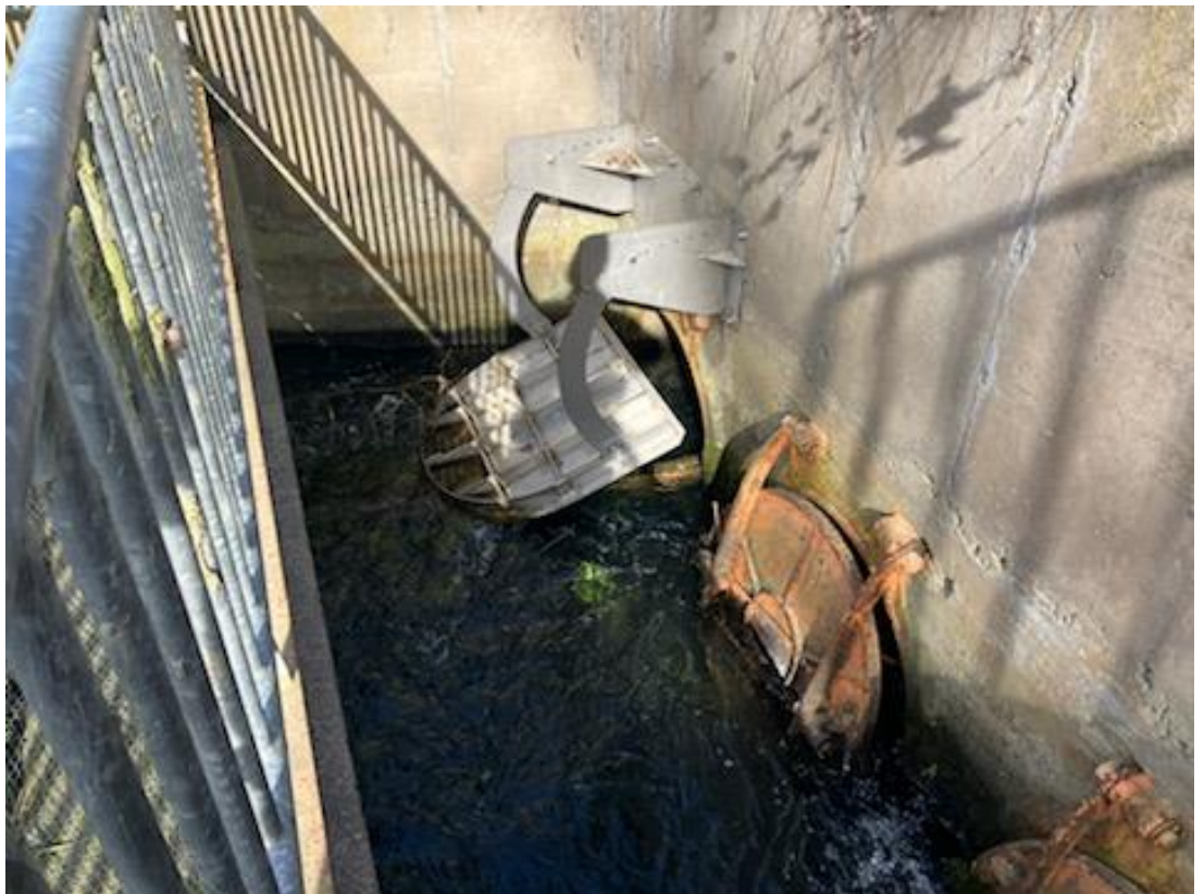
Photo 4 – Log stuck in flap valve
