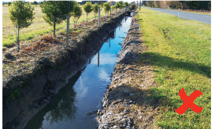
Herbicide spray causing unstable banks
