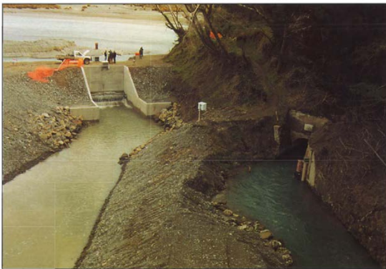
The new intake and the old tunnel (note the commemorative plaque). This tunnel is now registered as an "Historic Place". August 1999
