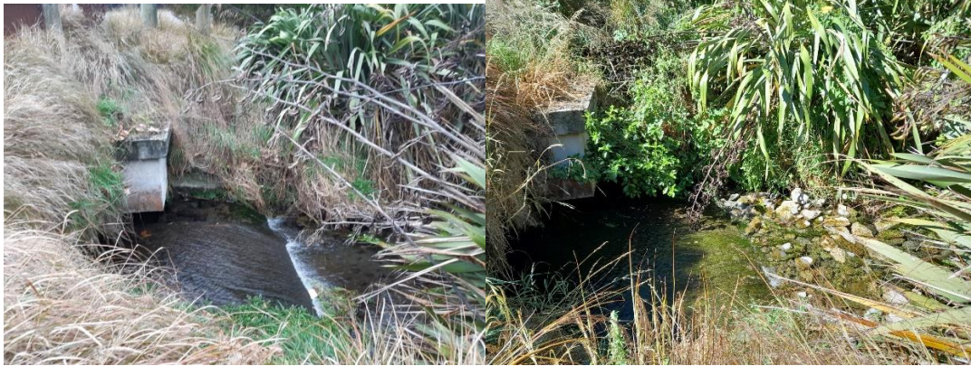
Figure 2: The likely fish passage barrier on a North Brook tributary – Corner of Cotter Lane and Northbrook Road before (left) and after (right) works were carried out
