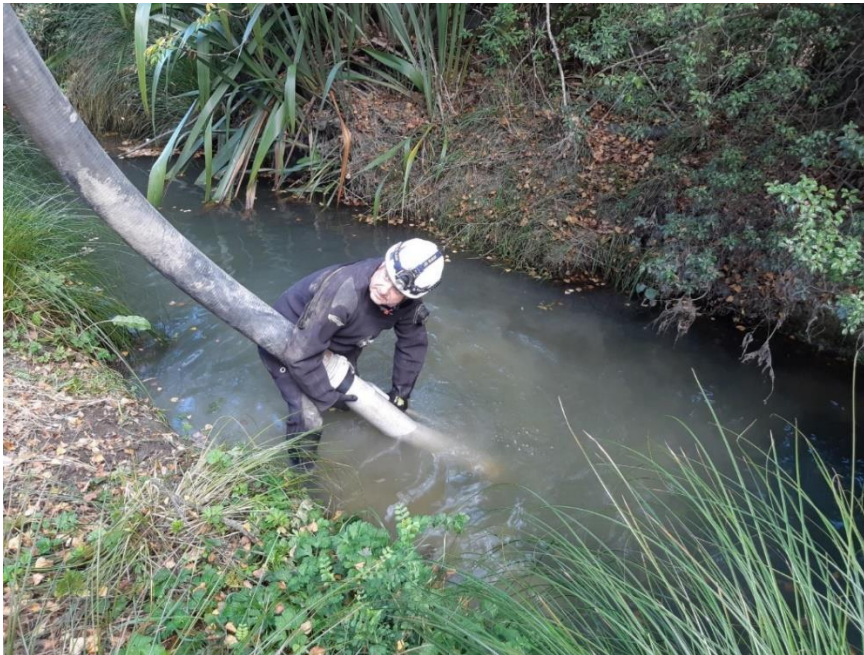
Figure 5 – The manual-handling technique for directing the vacuum suction pipe
