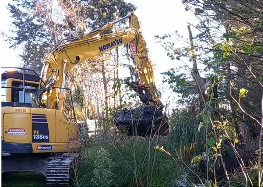
Figure 6: Removal of sediment from the Church Bush Road sediment trap on the Tuahiwi Stream / Waituere with a silt bucket
